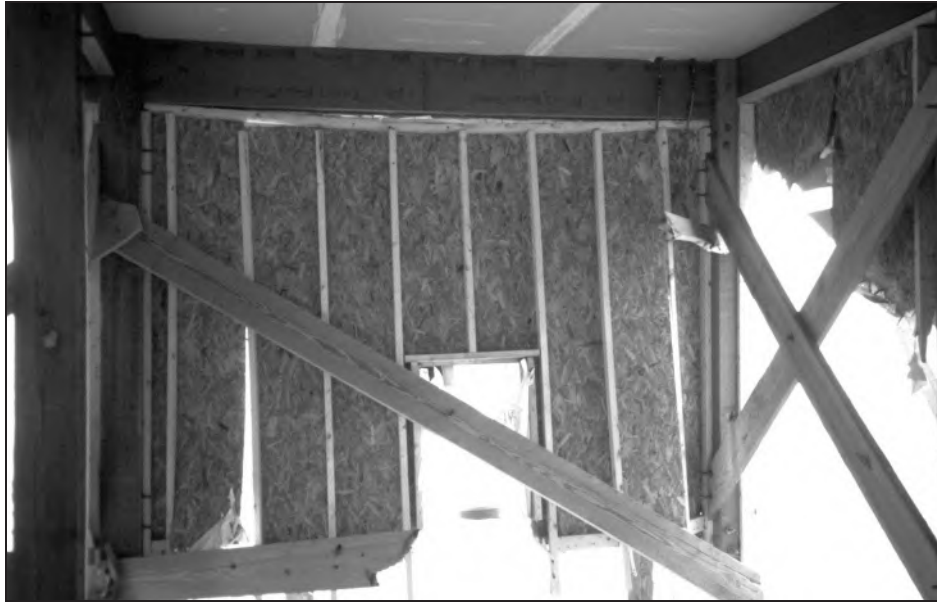
Figure 7. Non-compliant bracing arrangement
