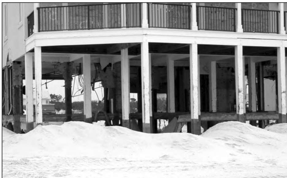
Figure 3. Successful breakaway wall performance
