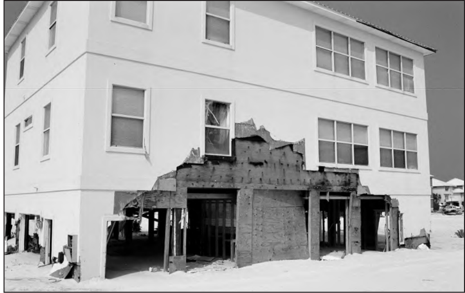
Figure 5. Non-compliant breakaway wall joint detailing
