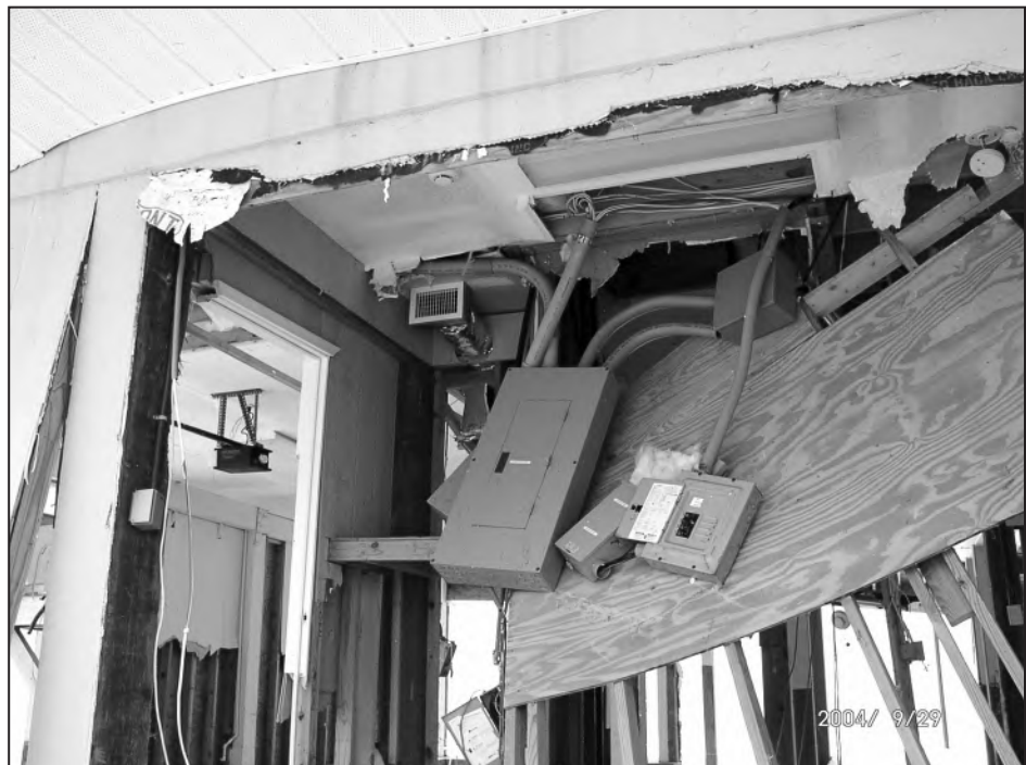
Figure 6. Non-compliant utilities attached to breakaway wall
