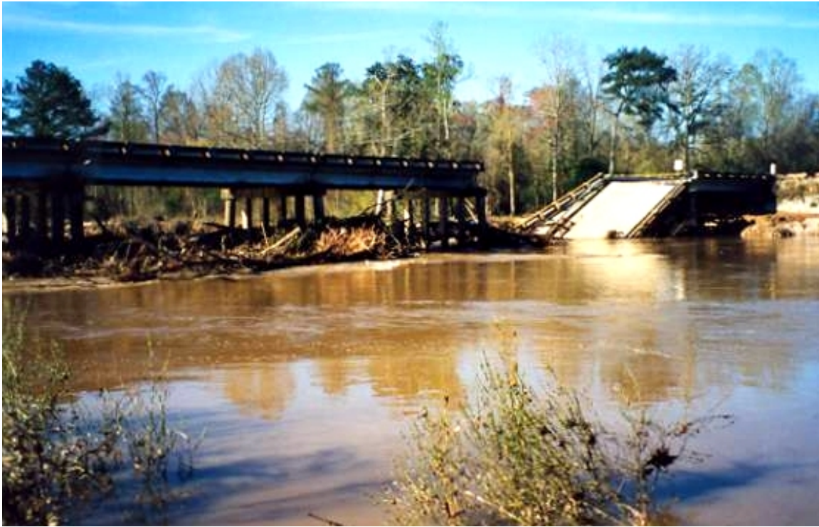
Figure 2.3. Span blockage accumulation bridge failure. (Louisiana)
