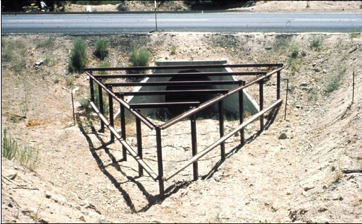
Figure 5.2. Steel rail debris deflector (looking downstream).
