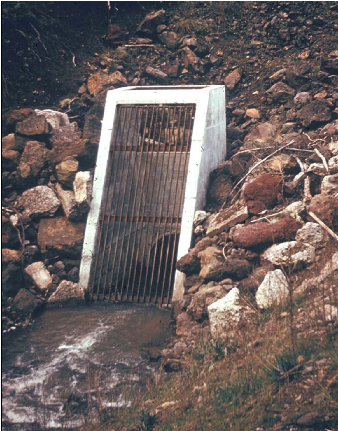
Figure 5.16. Debris rack used in State of Washington.
