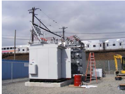
Fig. 25. 26/13 kV 9.0 MVA Unit Substation
