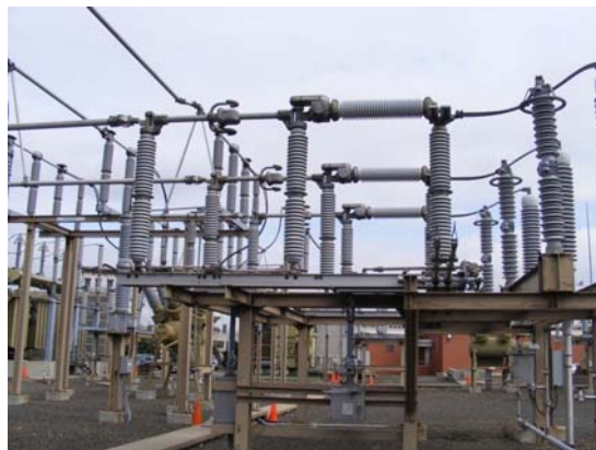
Fig.11. 230 kV 1200 A Circuit Switcher Substation Bus Systems
