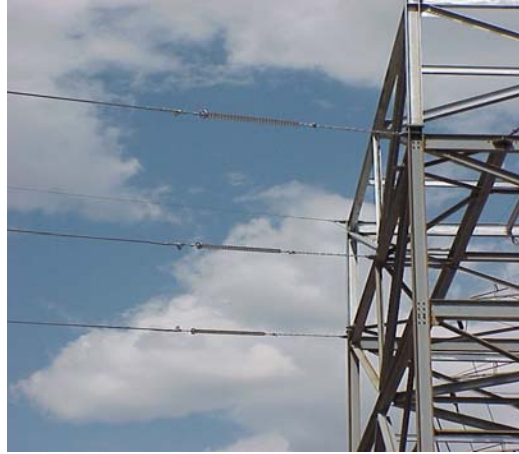
Fig. 15. 230 kV Strain Insulator Assembly
