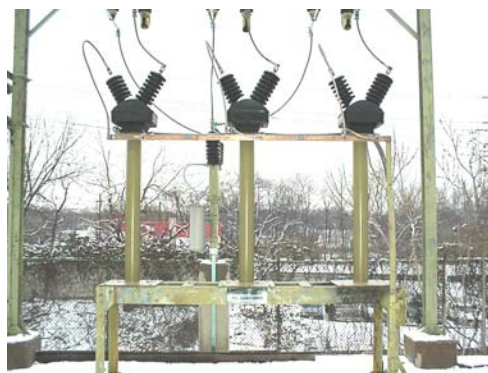
Fig. 21. 26 kV Potential Transformers
