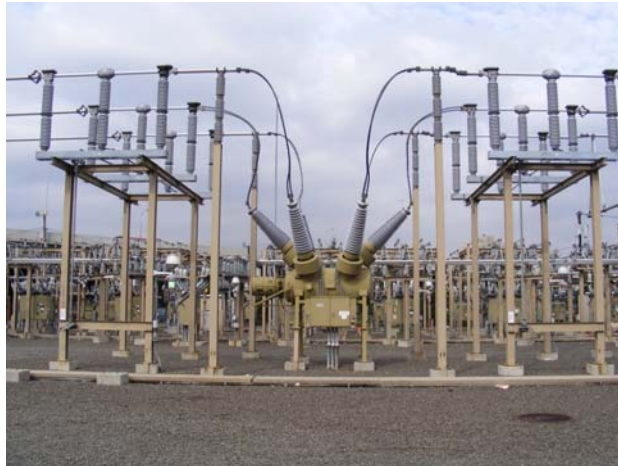
Fig. 5. 230 kV Outdoor 2000 A Circuit Breaker
