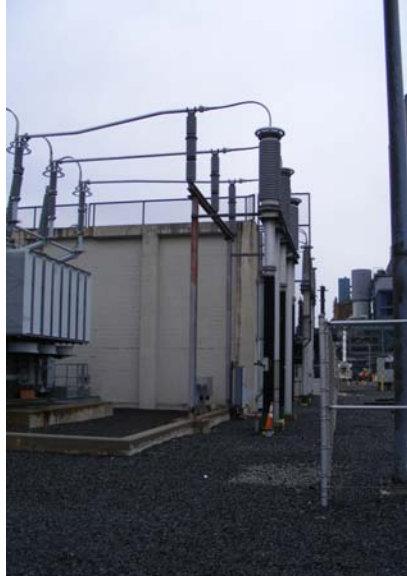
Fig. 16. 230 kV Gas Insulated Bus
