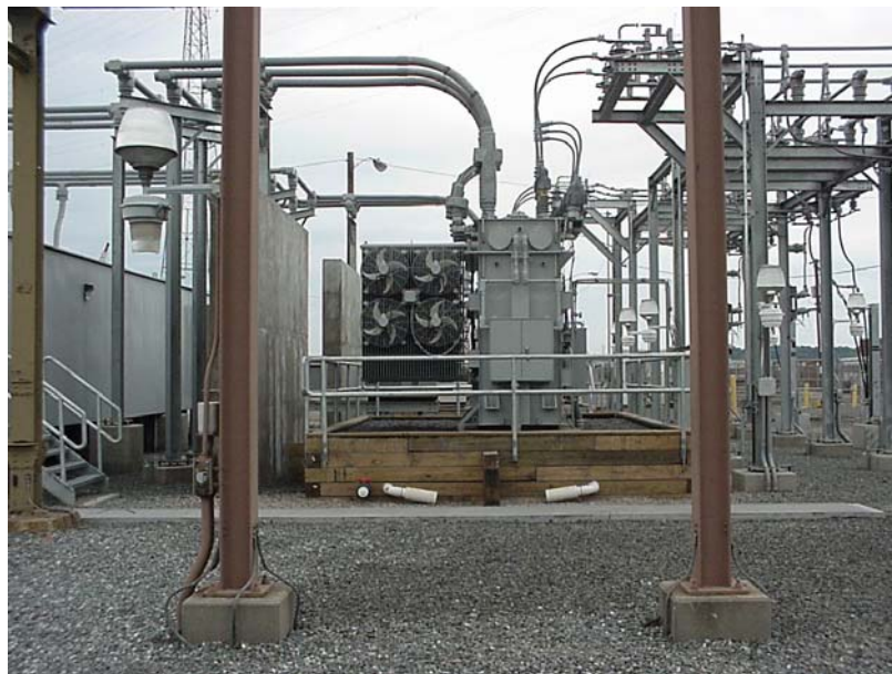
Fig. 3. 13/4 kV 6.0/9.0 MVA OA/FA Transformer
