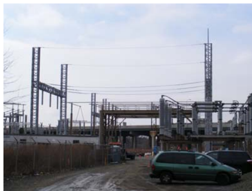
Fig. 14. 230 kV Strain Bus on Steel Towers
