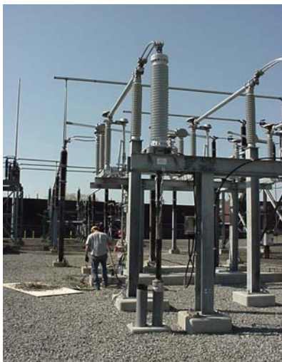
Fig. 17. 138 kV Solid Dielectric Cable Bus Terminal
