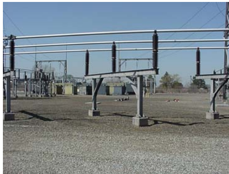
Fig. 12. 138 kV Open Air Bus on Post Insulators
