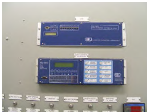
Fig. 2. Microprocessor Relays Installed on the Panel
