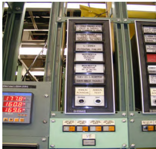
Fig. 19. 6- Window Substation Annunciator
