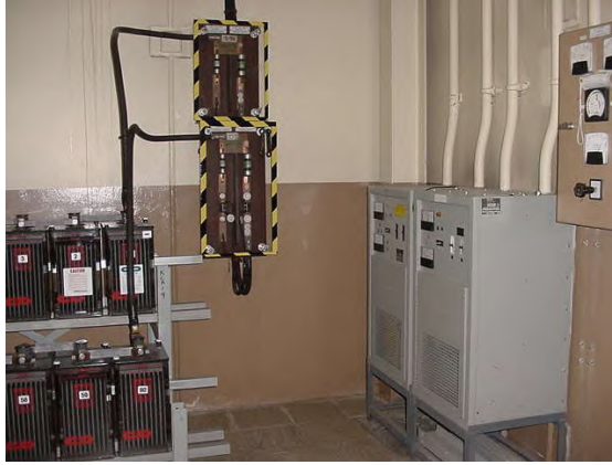
Fig. 18. Substation Auxiliary DC Equipment
