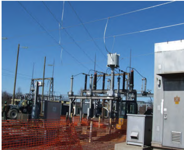
Fig. 12. 138 kV CCVT with 3000 A Wave Trap
