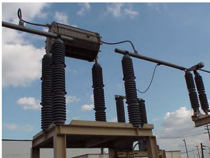
Fig. 13. Free Standing 138 kV 2000 A Wave Trap
