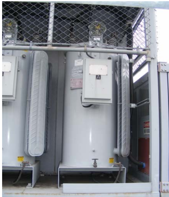
Fig. 14 - 4 kV Voltage Regulators
