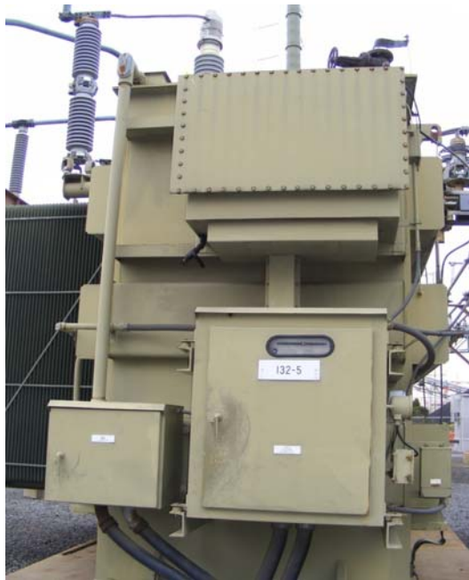
Fig. 13 - 26 kV LTC on 230/26 kV 55 MVA Transformer
