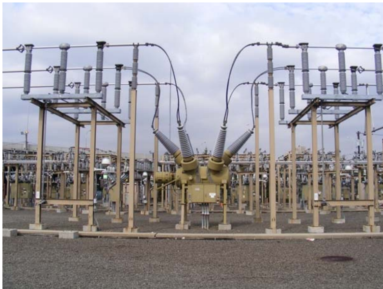
Fig. 8 - 230 kV 2000 A Circuit Breaker
