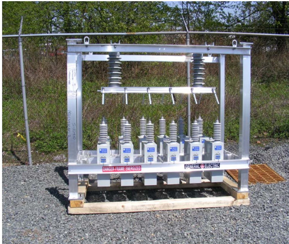
Fig. 4 - One Phase of 26 kV Capacitor Bank
