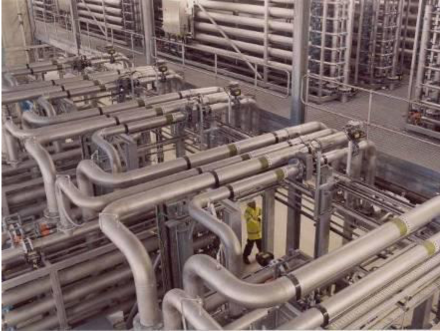
Clay Lane - London (UK) 6,700 m 3 /h
