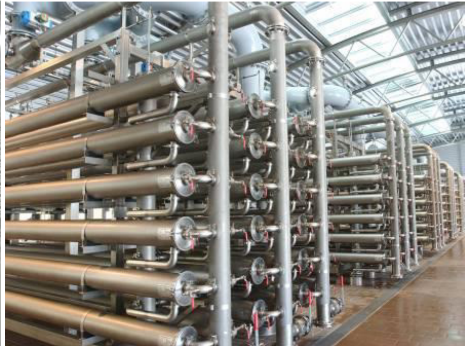
Roetgen (Germany) 6,000 m 3 /h
