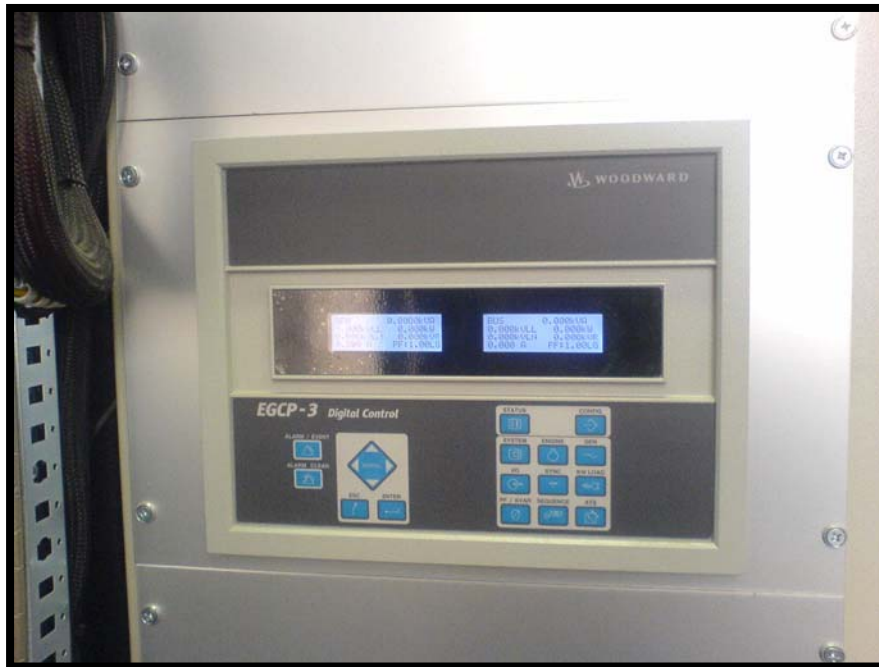
A pictorial view of Generator synchronizer
