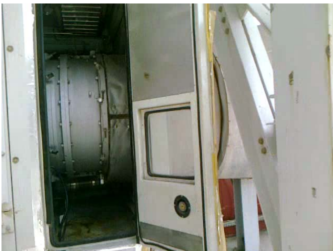
A view of the GTG exhaust
