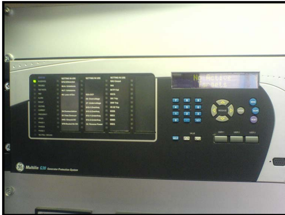
G30 Generator protection system
