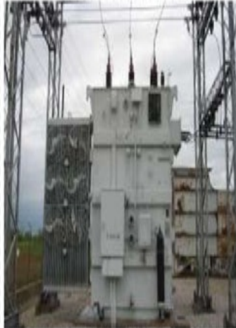
Step Up Transformer
