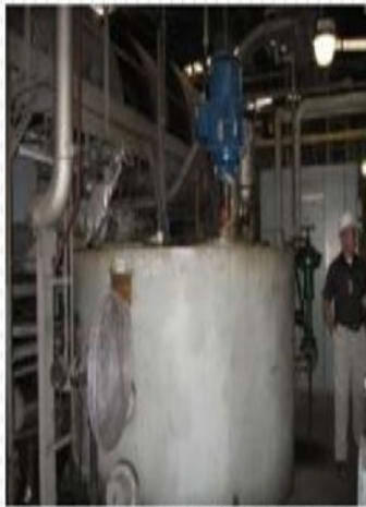
Lube Oil System
