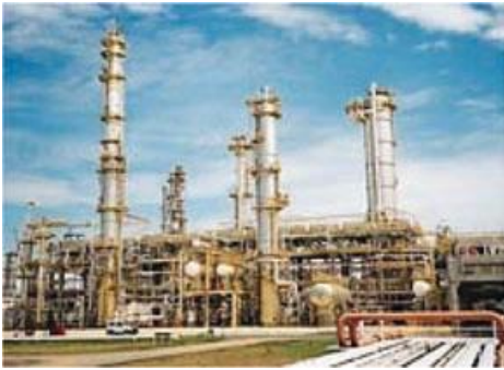
Fluid heating in a petroleum process heater
