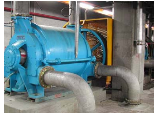
Figure 5: Example of vacuum pump
