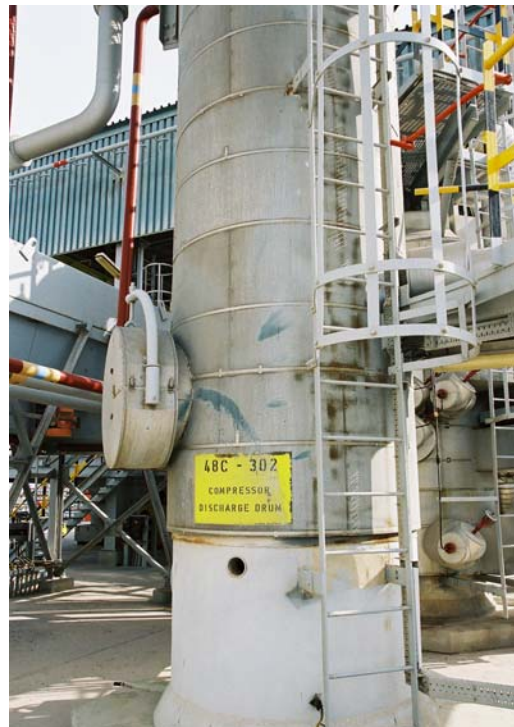
(b) Discharge Knockout Drum
