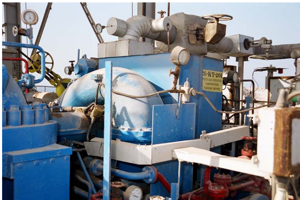
Figure 5.17: Steam Turbine Driver (Tag# 26-KT-101 and 201)
