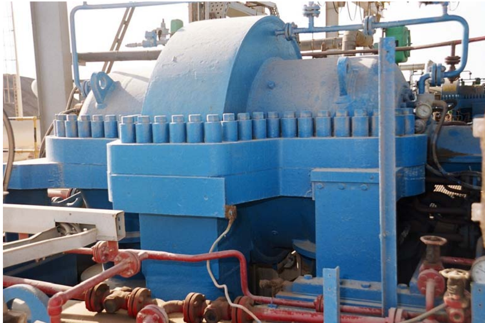
Figure 5.16: Booster Compressor (Tag# 26-K-101 and 201)
