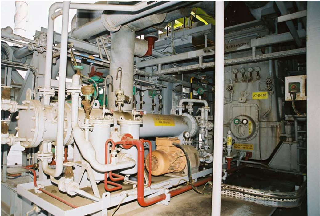
(a) Lube-oil Supply for VRU Compressor
