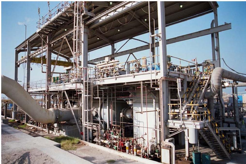
Figure 5.2: Booster Compressor Platform, Trains I and II
