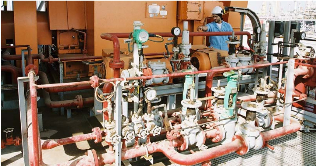
(b) Lube-oil Supply for New BOG Compressor
