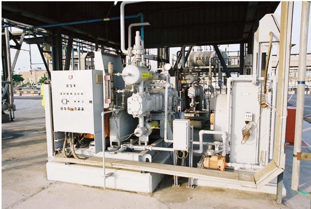
Figure 4.2: STOREX Air Compressor (Tag# 28-K-70)
