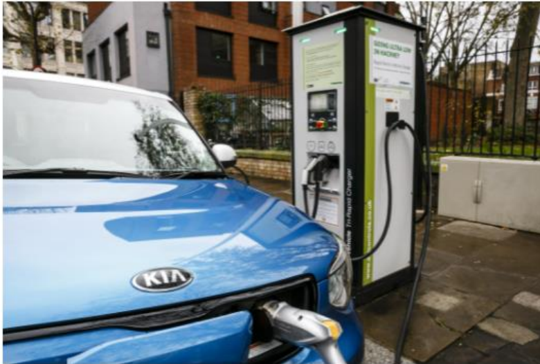
Level -2 Charging (EVSE)
