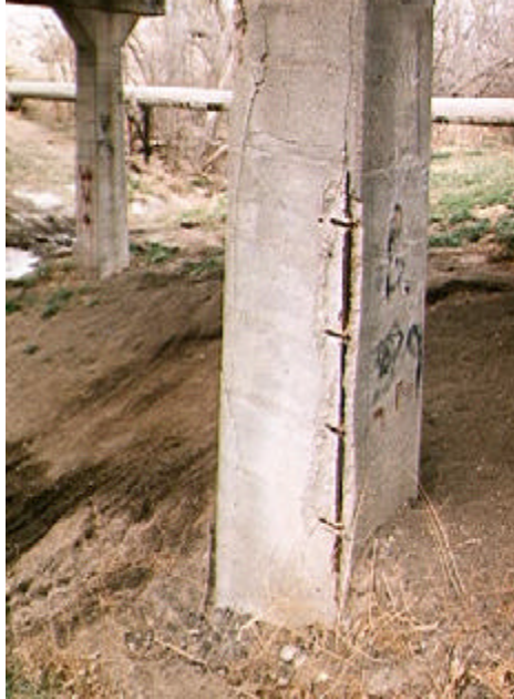
Figure 1. Corrosion-induced deterioration on a bridge column.
