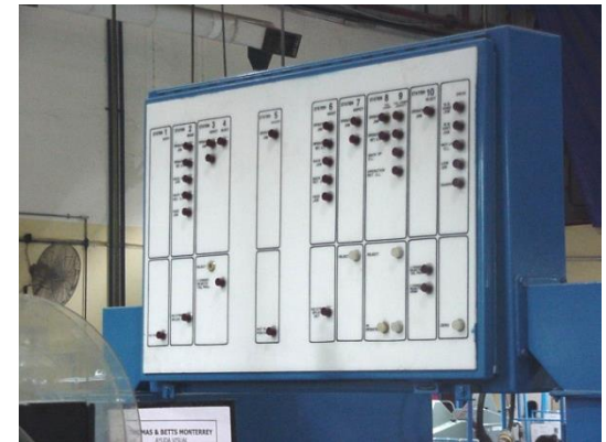
Lights connected to Micro switches & timers
