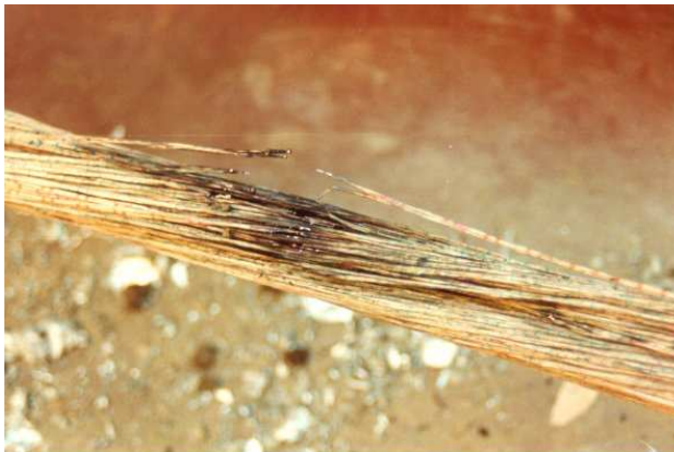
Photo 2: Damaged Telecom Cable
