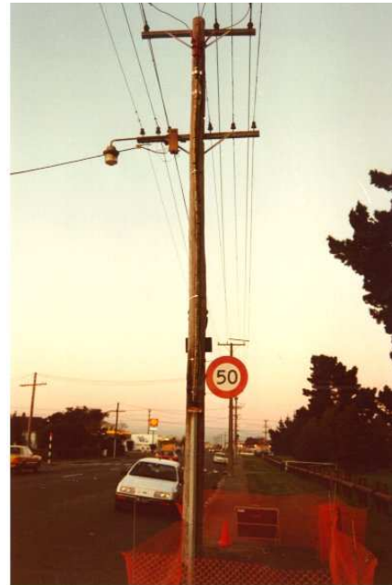
Photo 3: 11 kV Cable on Pole
