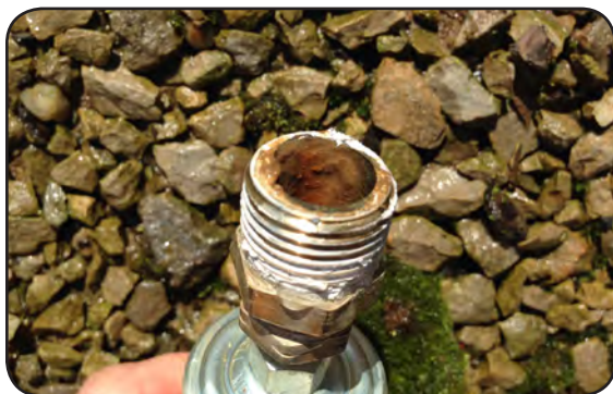
Figure 17. Sediment in Irrigation lines
