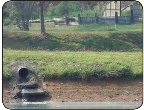
Figure 1. Irrigation pond below desirable water level
