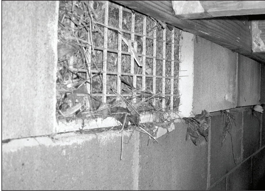
Figure 15. Typical air vent clogged by flood debris
