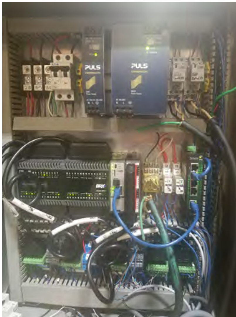
Figure 8i: Control Panel: This new AutomationDirect BRX PLC replaced the existing Click controller with minimal required changes or wiring additions.
