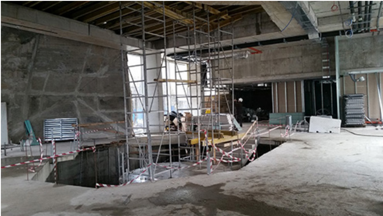
Figure 8D: Bat Exhibit under construction at the Children's Center of Sofia, Bulgaria.
