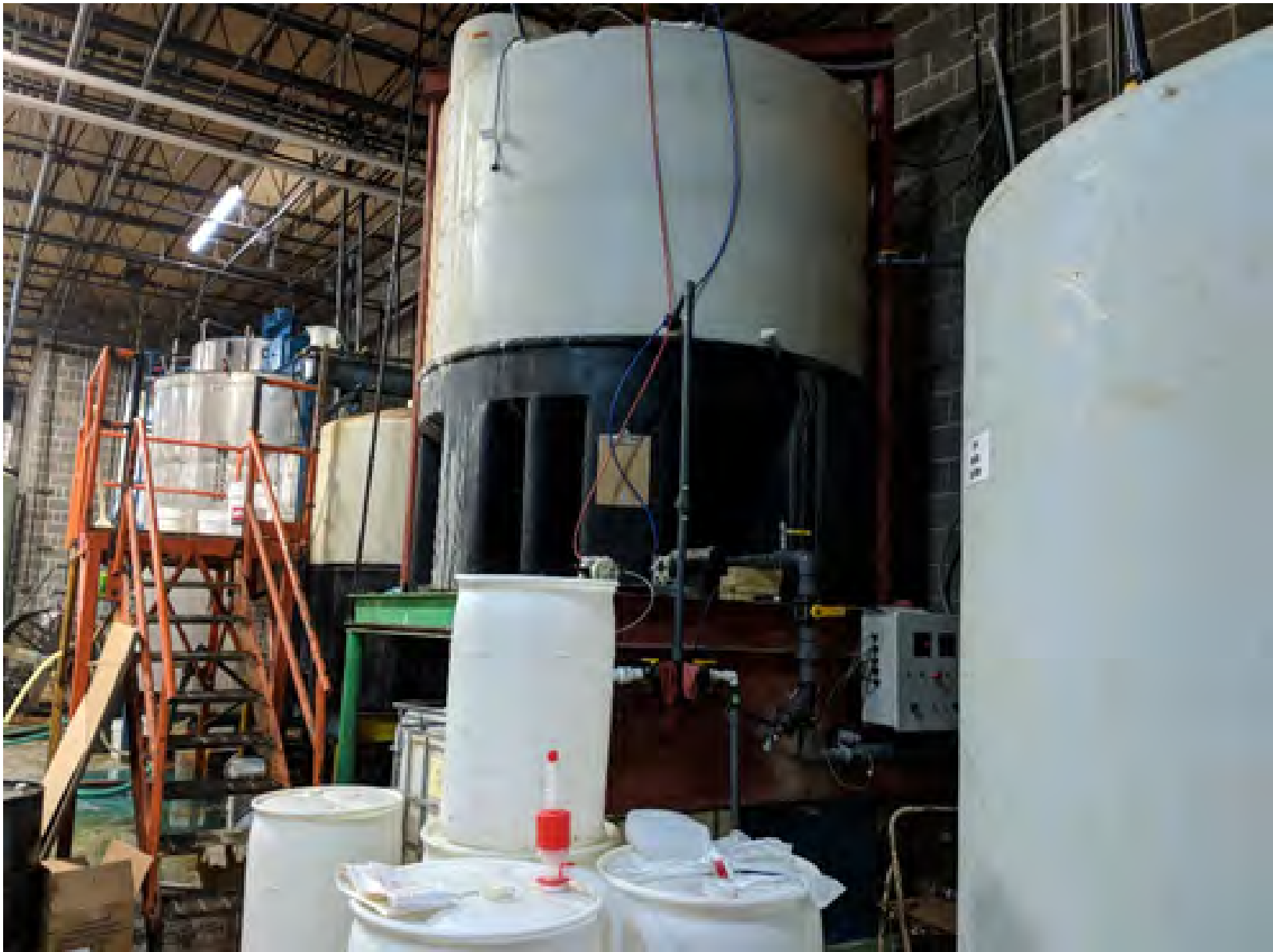
Figure 8H: Acid and caustic tanks: These tanks hold the acid and caustic needed to balance the PH of the wastewater produced from a large agriculture components metal coating process.
