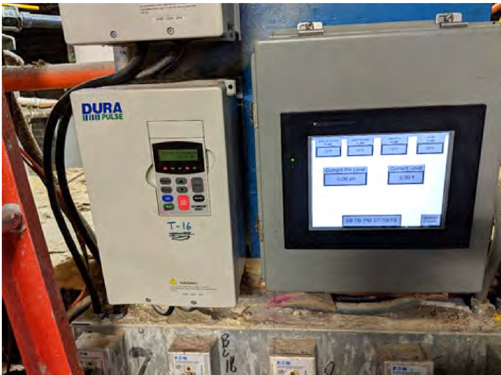
Figure 8J: HMI: An AutomationDirect C-more EA9 Series 15-inch touch panel HMI was added to the new control system to provide status, data trending, historical data, reporting and other functions.
