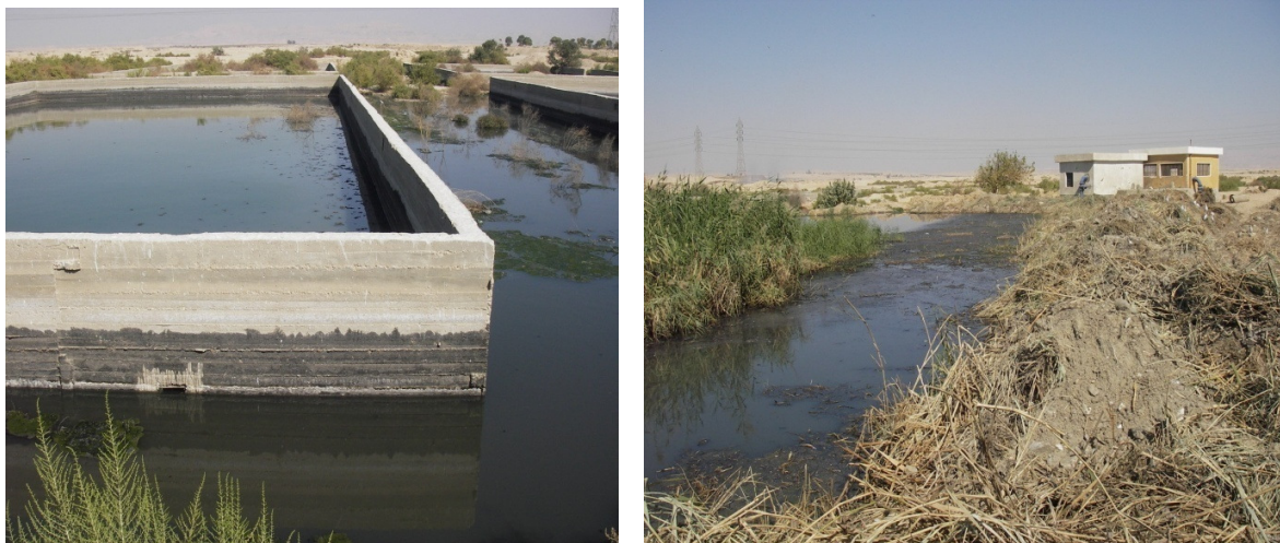
Figure 13: Buffer bonds with pump station (left) and outflow by gravity (right) Source: GAIA-Tec, Jan 2008
