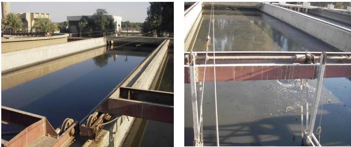
Figure 9: Sludge scrapers (out of service) Source: GAIA-Tec, Jan. 2008
