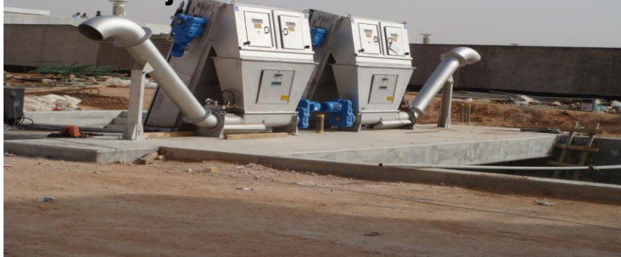
Complete screening Inletwork of Al-Kharj k29 STP 2008
