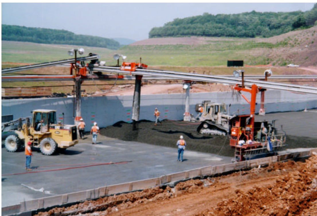
Figure 6-2. Conveyor system with mobile side discharge belt
