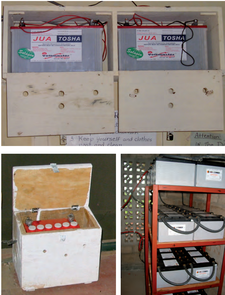
Figure 9.10 Battery box, rack and shed
