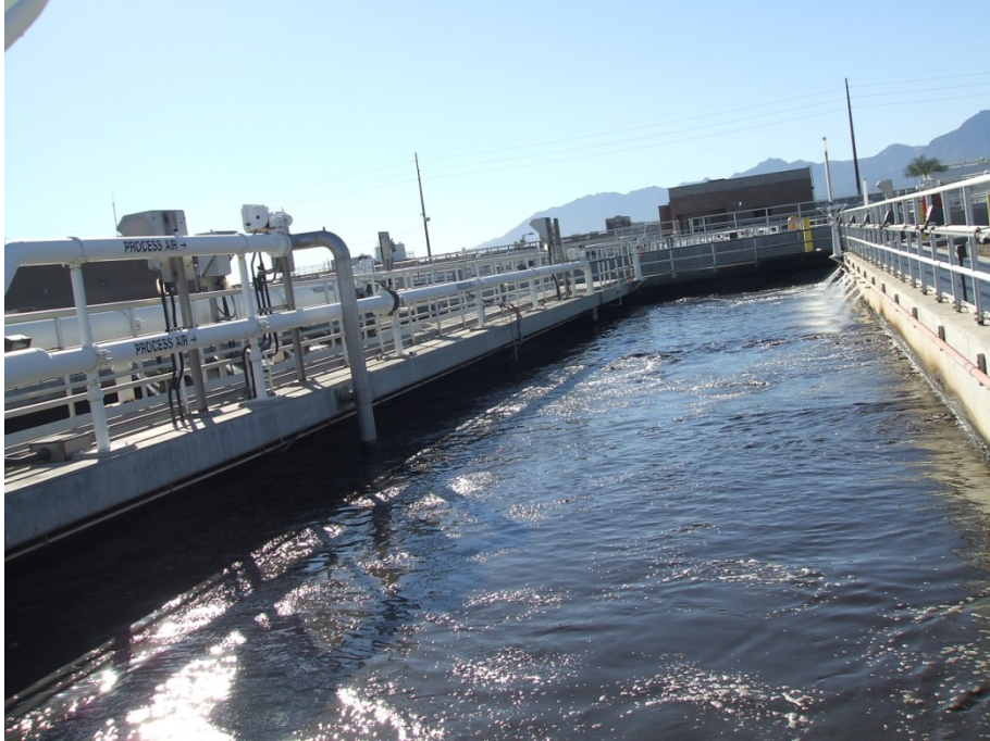
Anoxic zone, denitrification area.
