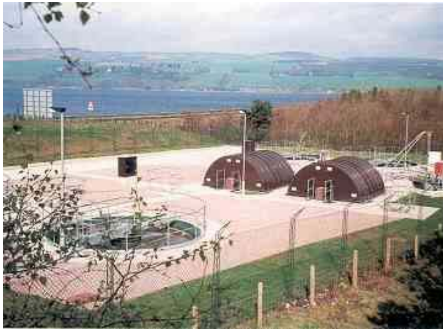
The recently completed installation at Culbokie, for Scotland Water.
