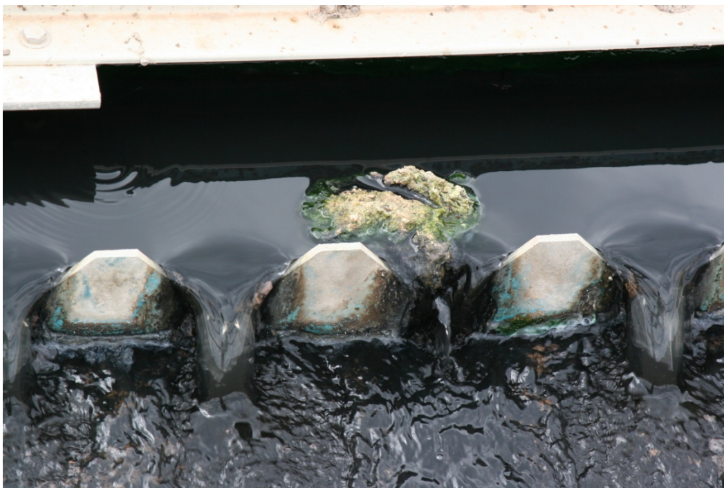
Caked grease stuck on weir.
