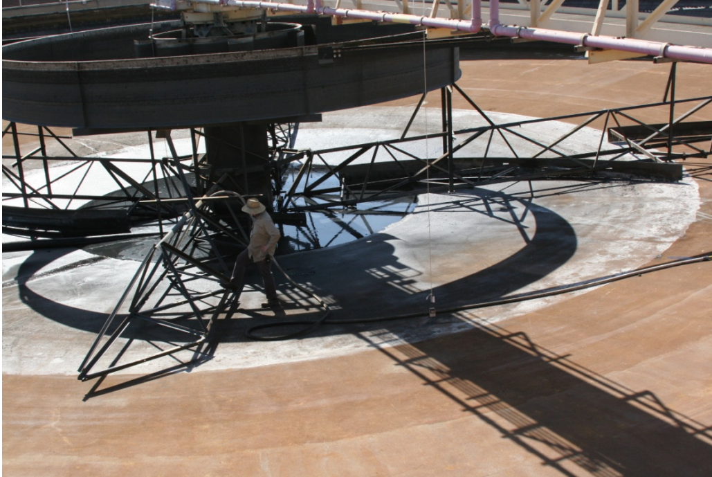
Scraping mechanism inside a clarifier.
