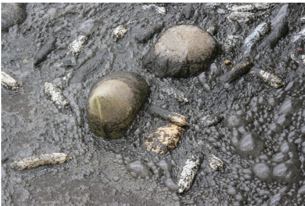
Floating scum in primary clarifier.
