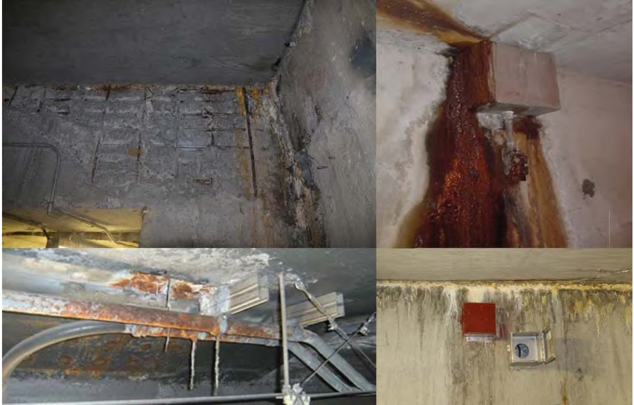
Figure 3.1 – Groundwater induced corrosion and deterioration.
