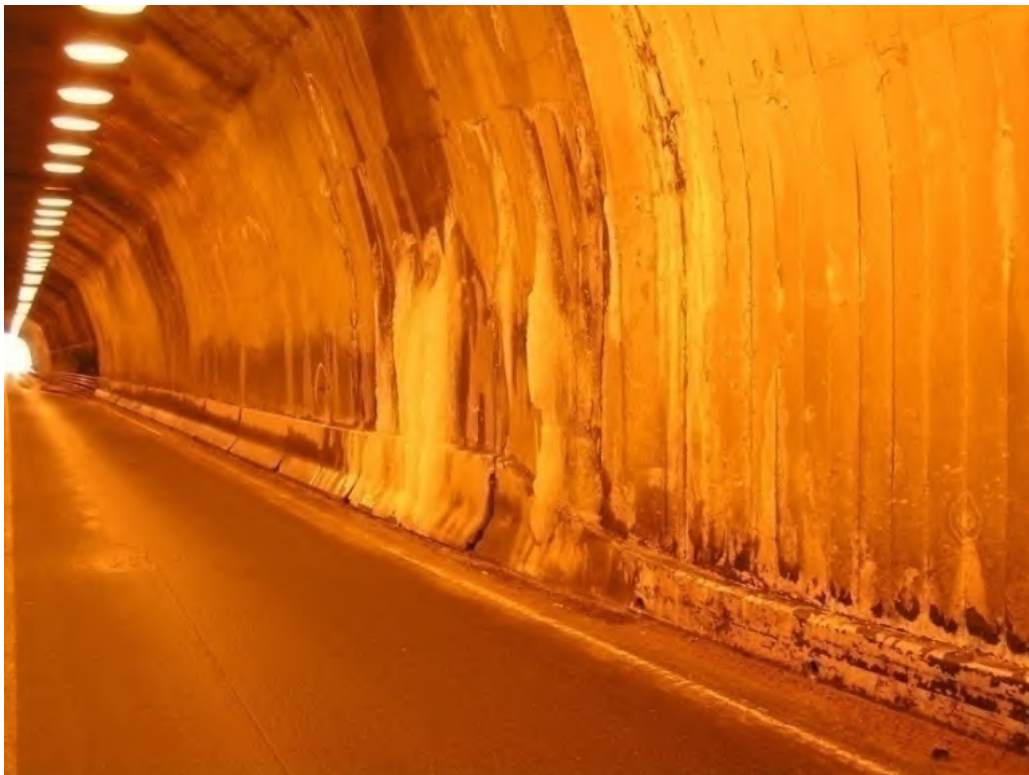
Figure 3.2 – Leakage through shotcrete liner (NCHRP, 2010).
