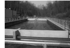
SBR – Sequencing Batch Reactor
