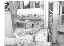
Mechanical bar screen with debris
