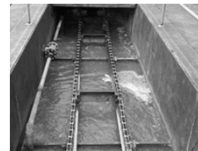
Aerated grit chamber
