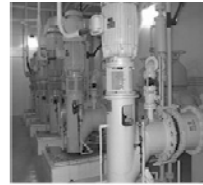
Raw wastewater pumps, Ames, IA
