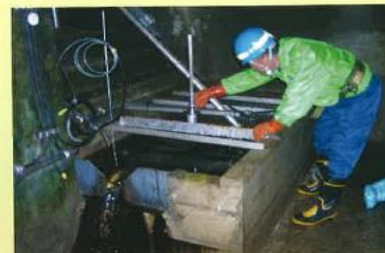
Photo-30 Measurement of Leak
