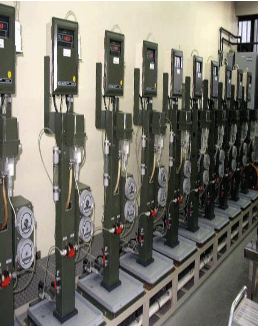
Residual chlorine meter
