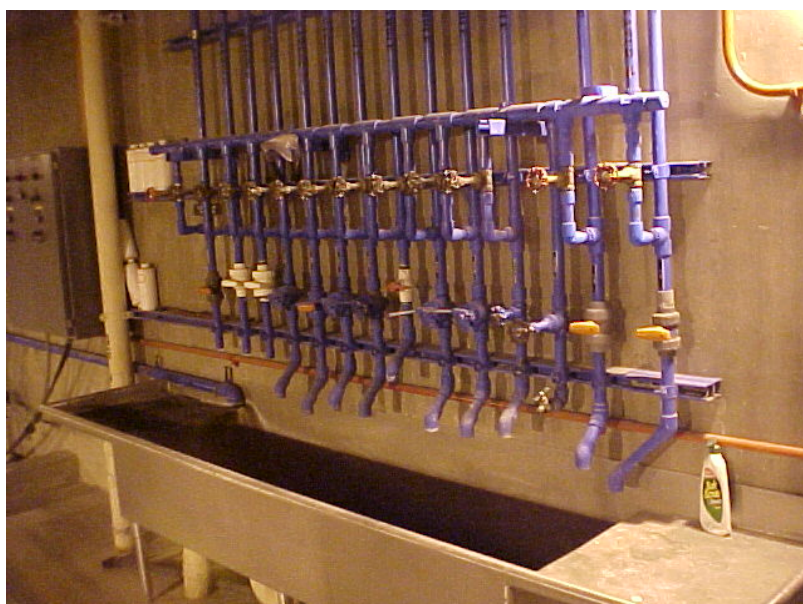
Sample taps inside a Water Treatment Facility
