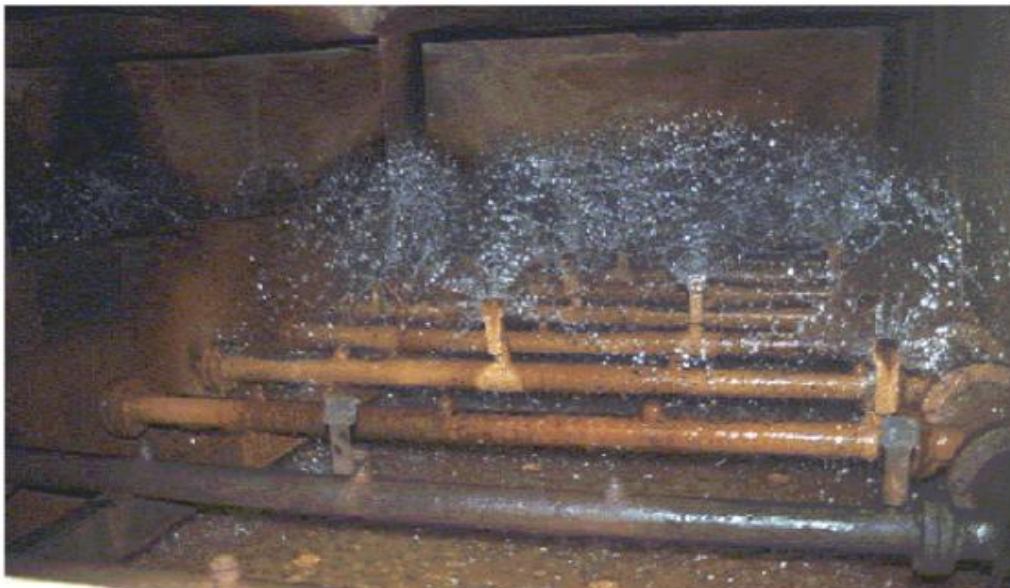
Figure 4 - Aeration above limestone filter
