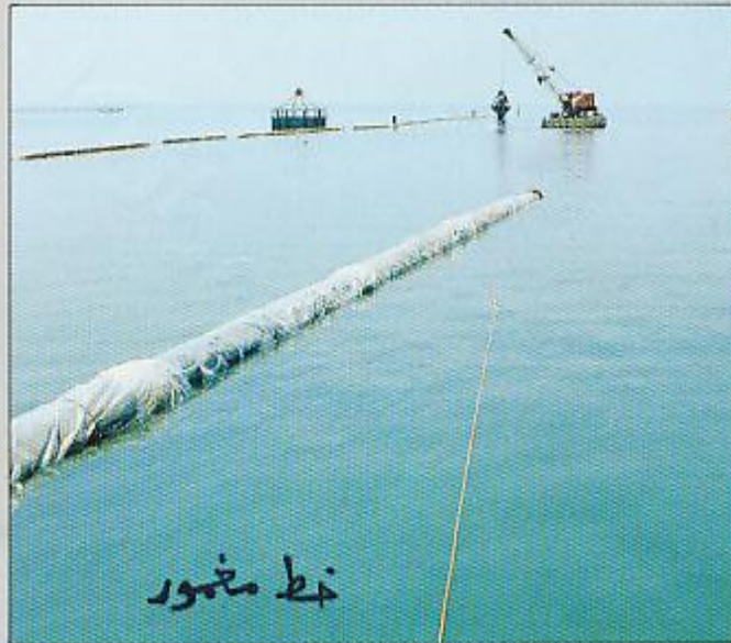
Sewage pipeline (Submerged piping)
