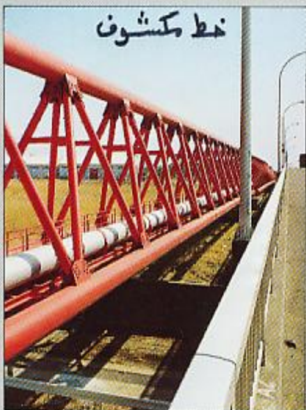
Water supply pipeline (Water-bridge piping)
