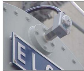
Bladder Failure Relay
