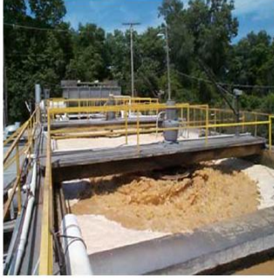
Aeration by Aerator
