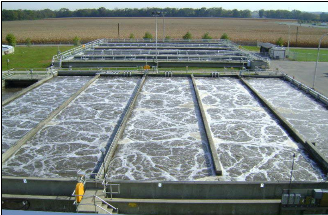
Figure (2.9-b): Aeration Tanks in an Activated Sludge Treatment [9].
