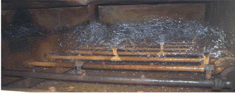
Figure 4 - Aeration above limestone filter
