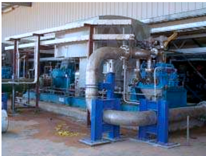
Figure 4. Largest Pelton Wheel energy recovery system in the world (Trinidad)
