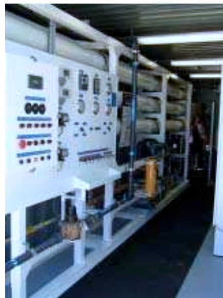
Figure 7. ADC Seawater Desalination Facility (Pt. Hueneme, California)
