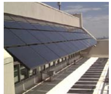
Inclined PVs with windows
