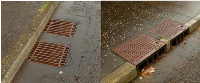
Figure 1. Examples of typical storm drain inlets.
