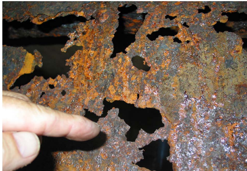
General corrosion - Structural steel I-beam support
