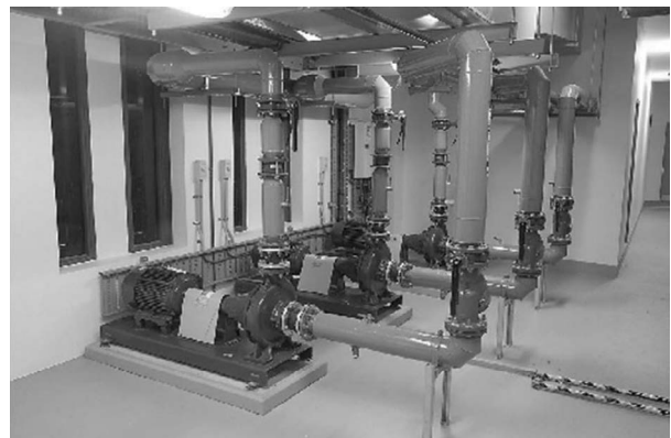
Figure 7.42. Cooling water pumps are often installed parallel to each other.
