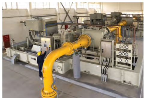
Figure 7-6. Electric-motor drive package: VFD controlled motor driving the compressor via a speed-increasing gearbox.
