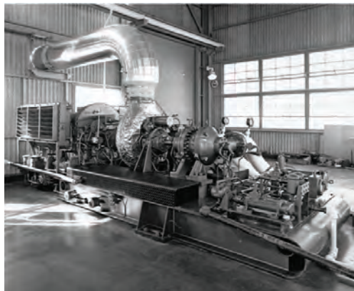
Figure 0-4. Solar Saturn gas turbine driving a C16 compressor (ca. 1961).
