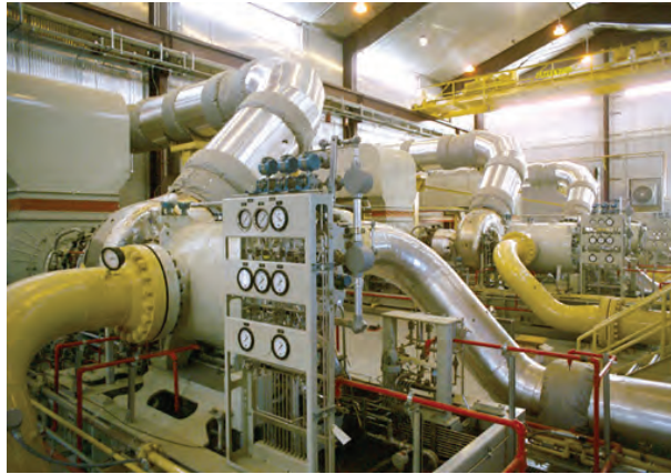
Figure 8-21. Pipeline compressor station with three compressor trains in parallel.
