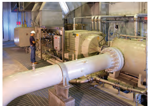
Figure 7-5. Electric-motor drive package: constant-speed motor driving the compressor via a variable-speed gearbox.
