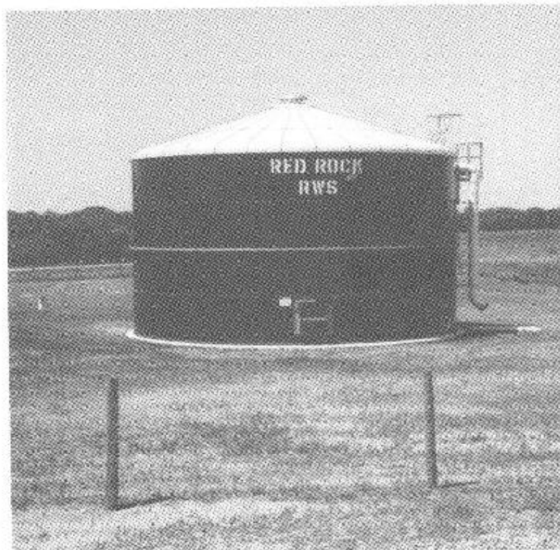
A Ground Storage Tank
