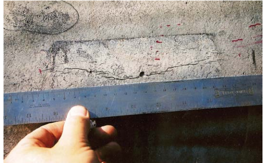
Sample pipeline stress corrosion cracking. (Schraan)
