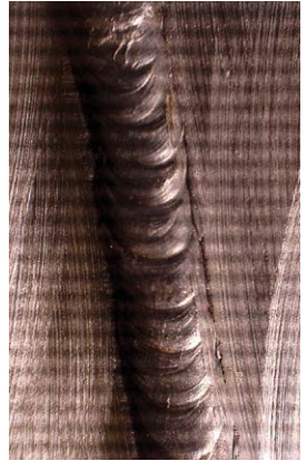
Inside diameter root crack. (Sabolik)
