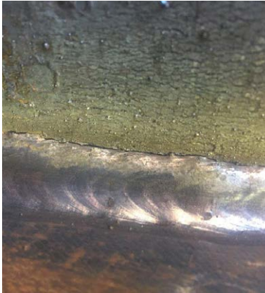
Outside diameter delayed toe crack. (Freeman)
