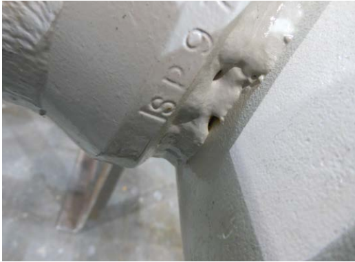
Underfill, porosity, and lack of fusion. (Wright)
