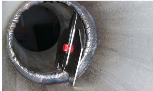
Excessive ID penetration. (Wright)
