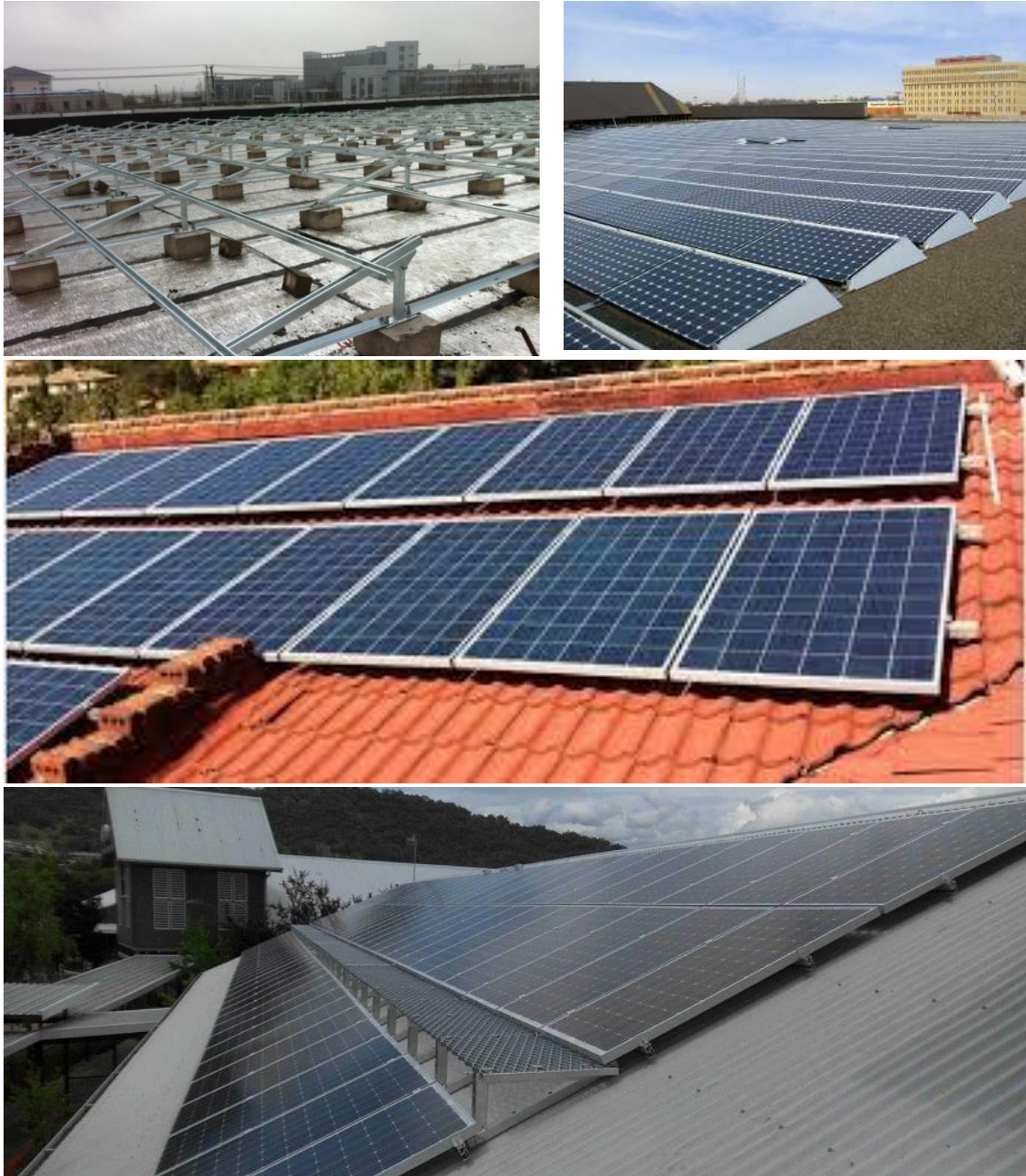
Figure 15: Different Rooftop Array Mounting Structures
