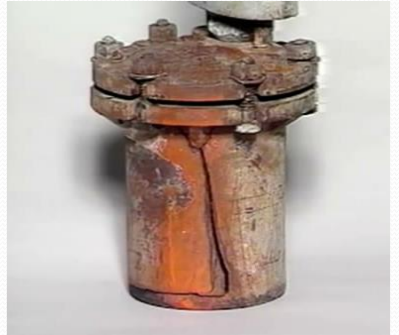
burst piping or damage
