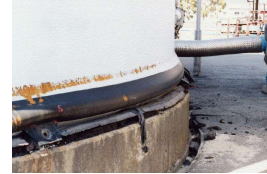
(c) Elephant foot bulge type buckling of tank wall
