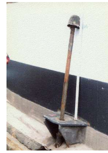
(a) Pulled out of anchor bolt
