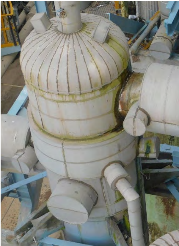
Figure 4. Degraded cold insulation.
