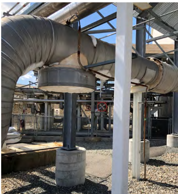
Figure 6. Icing on cold insulation.
