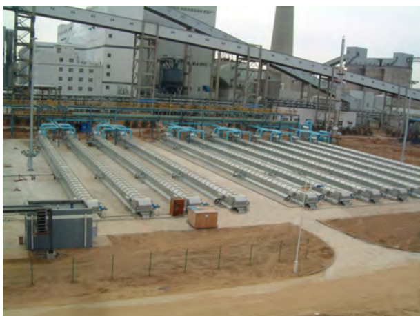
Figure 4. IPCO's pitch solidification plant.
