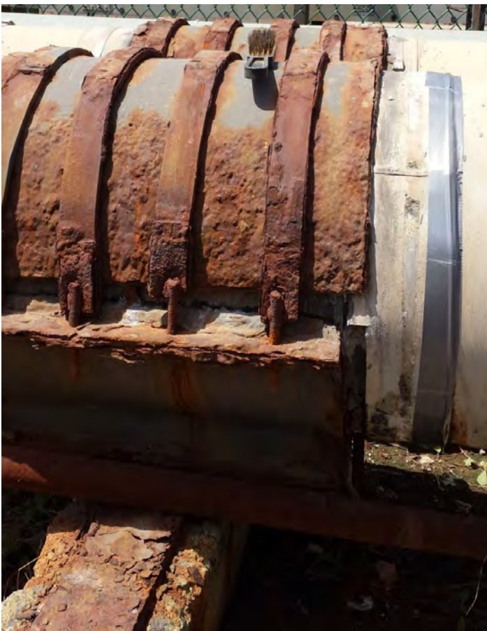
Figure 5. Rusted pipe supports.
