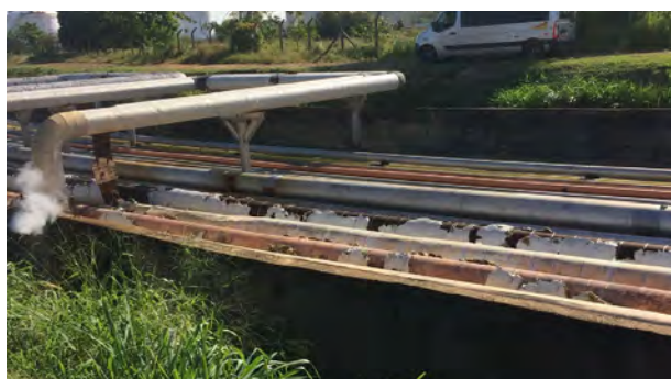
Figure 3. Degraded hot insulation.
