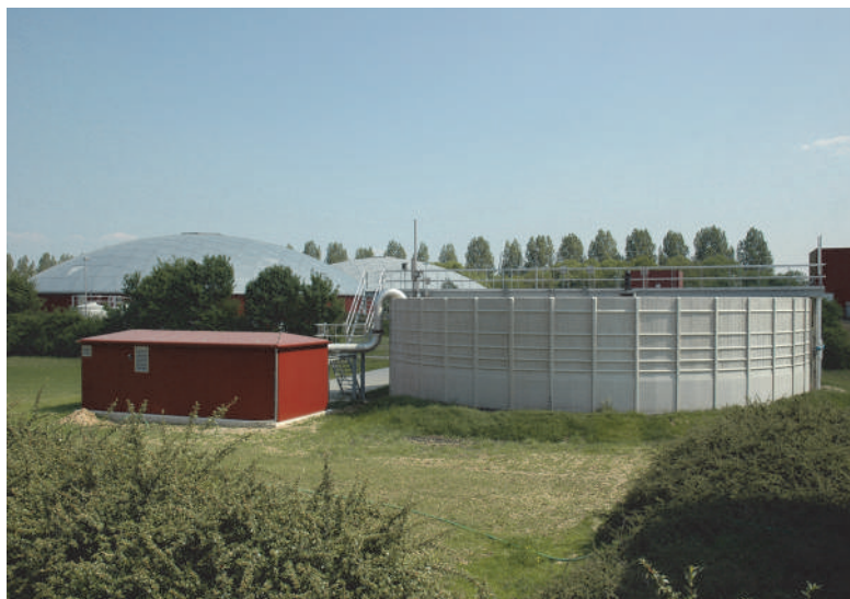
Figure 5.33 Full-scale application of the BABE ® technology: WWTP 's-Hertogenbosch in the Netherlands (at the front is the bio-augmentation reactor; photo: Royal HaskoningDHV).
