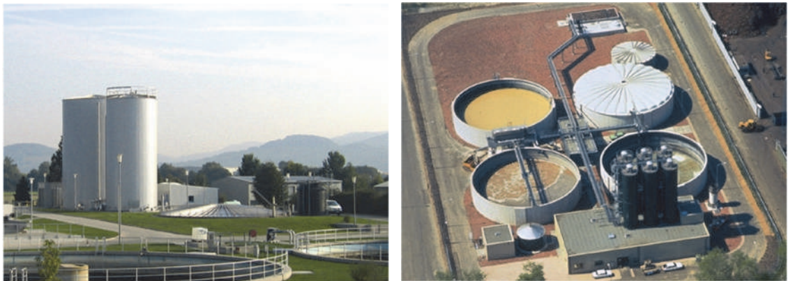
Figure 16.20 An EGSB installation for treatment of dairy wastewater in Germany (left) and an IC installation for treatment of brewery wastewater in Den Bosch in the Netherlands (right) (photos: Biothane B.V. and Paques B.V., respectively).
