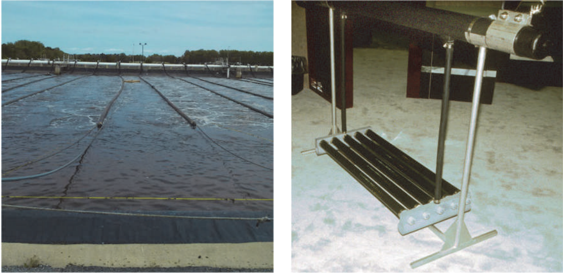
Figure 9.7 Fine-pore diffuser application in an aerated lagoon. The air pipes (on top of the diffuser unit) distribute the air along the lagoon, and vertical hoses convey the air from the air pipes to the diffuser units (placed close to the lagoon bottom). The image on the right shows a diffuser unit at a trade show. This system can be used in lagoons with uneven depths.
