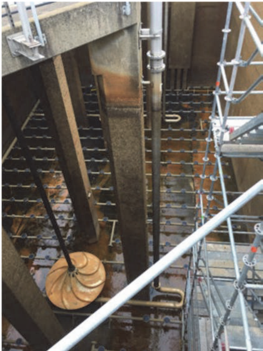
Figure 9.24 Pictures of the hyperbolic mixer deployed at a WRRF, installed above the existing diffuser grid.
