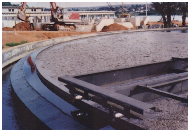
Figure 4.15B Rising sludge due to denitrification in the SST at one of the wastewater treatment plants in Brasilia, Brasil (photo: M. Henze).
