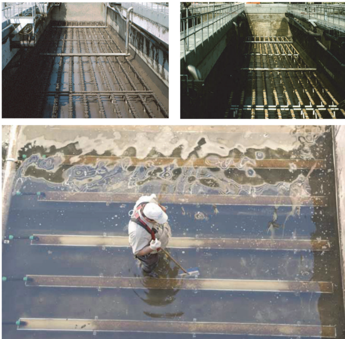
Figure 9.32 Examples of diffuser cleaning. Top: a dewatered tank equipped with ceramic domes before (left) and during (right) cleaning by means of tank-top hosing; the cleaned diffusers are clearly lighter in colour. Below: cleaning of polyurethane membranes by means of brushing.
