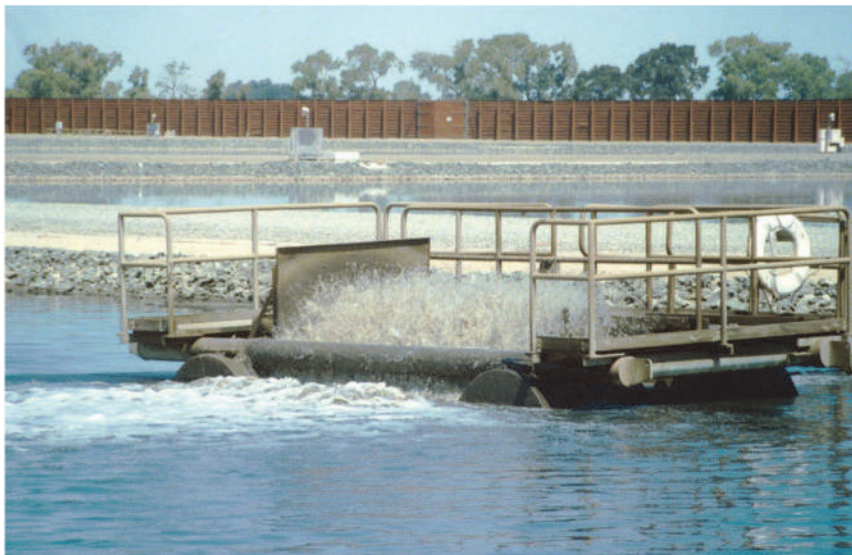
Figure 9.11 A surface brush aerator mounted on a barge in an aerated lagoon.
