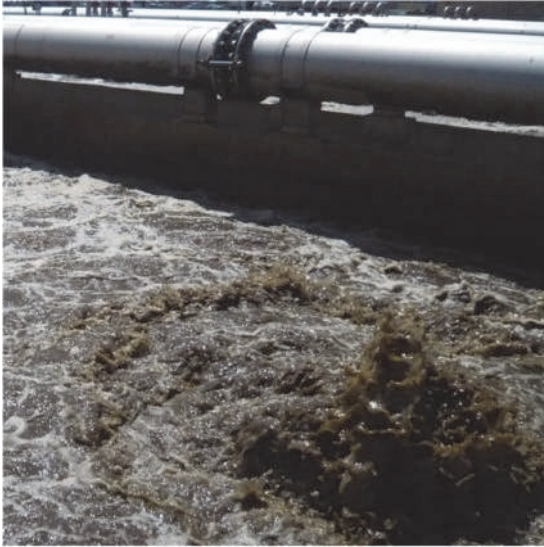
Figure 9.41 Surface boil indicating on the surface that at the bottom of the tank a diffuser is either damaged or an air header is leaking.
