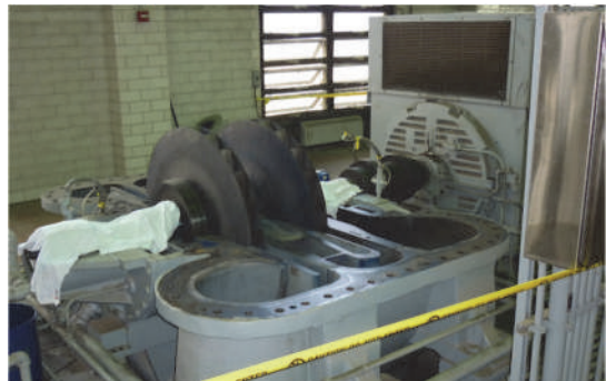
Figure 9.15 Multi-stage centrifugal blower schematic (top) and example of a multi-stage centrifugal blower in operation at a large wastewater treatment plant (second top). Below is a similar unit but during maintenance.
