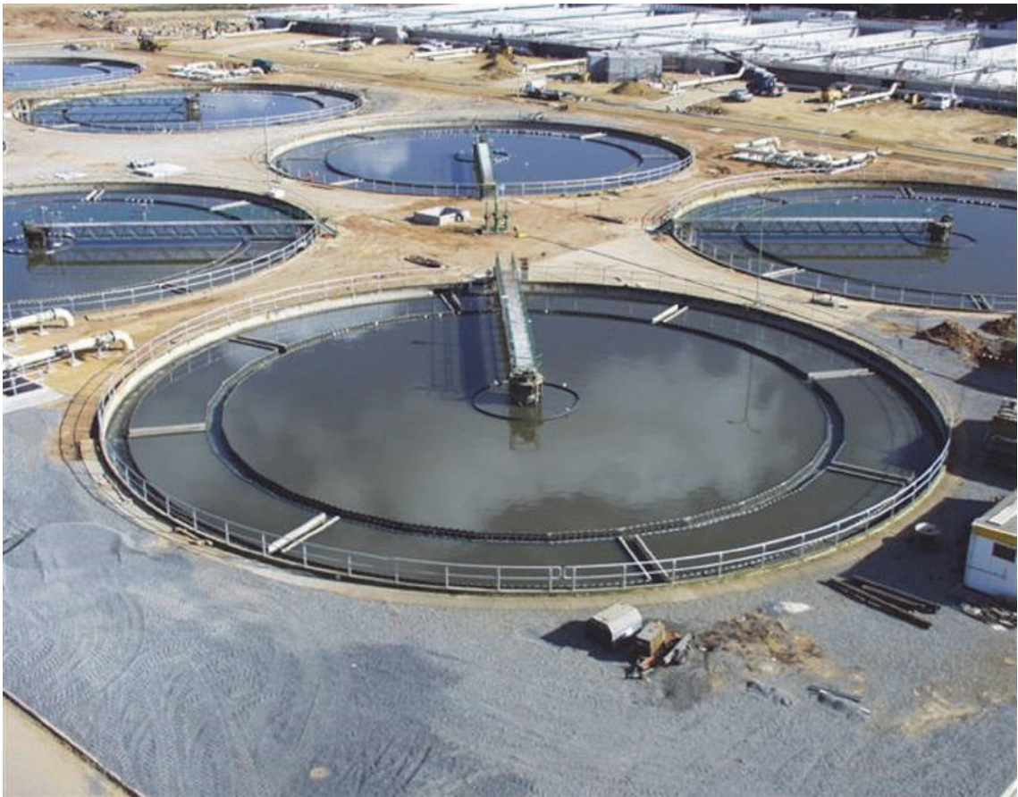
Figure 12.2 Circular clarifier (photo: EnviroSim).
