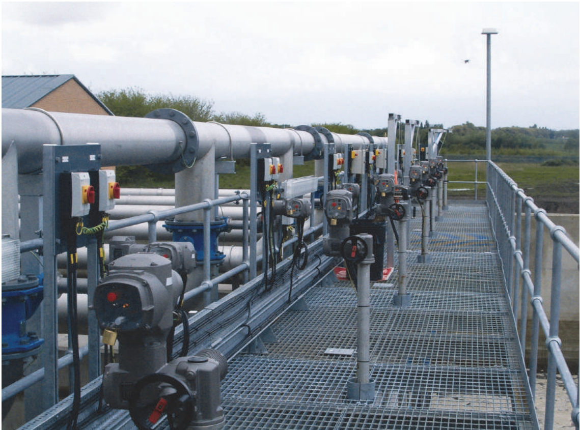
Figure 15.16 Detail of measuring and control system of activated sludge aeration tank (photo: D. Brdjanovic).
