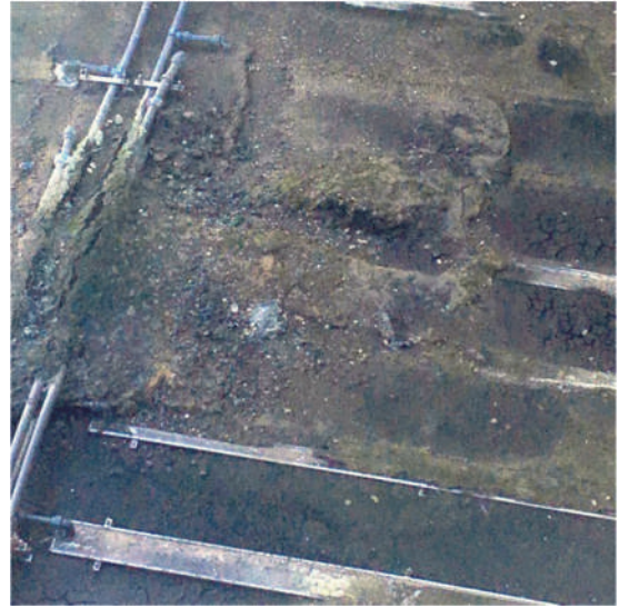
Figure 9.46 Example of the deleterious effects of grit accumulation on the aeration tank floor, with corresponding obstruction and damage to the diffusers.
