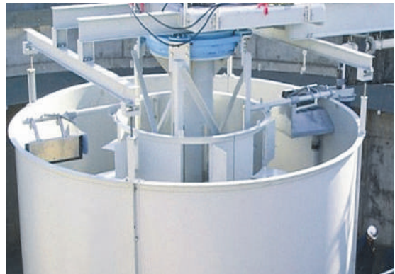
Figure 12.7 Flocculation well (photo: Brown and Caldwell).
