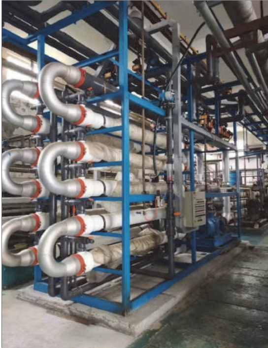
Figure 13.27 Membrane modules in the leachate treatment plant in Suzhou.
