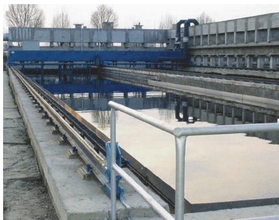
Figure 12.4 Rectangular clarifier (photo: D. Brdjanovic).
