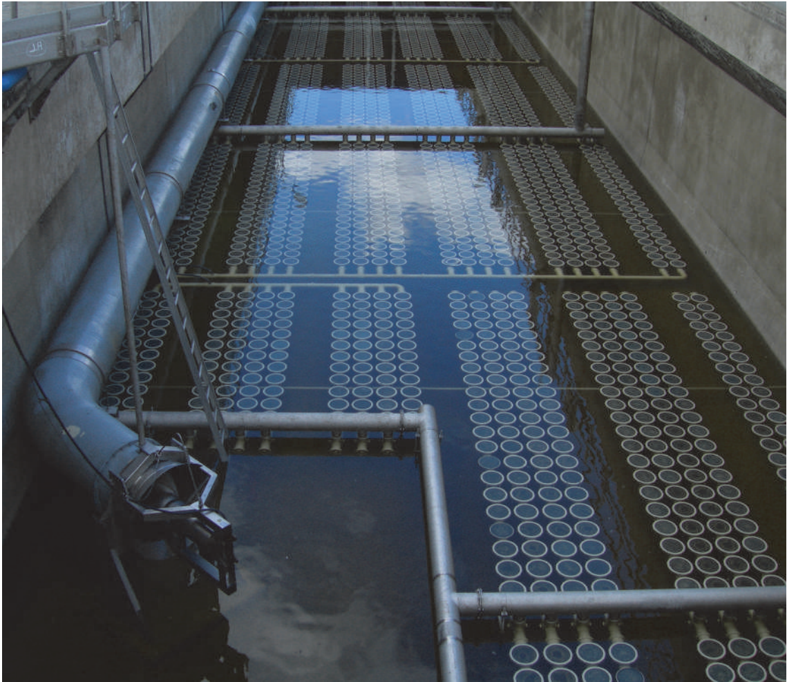
Figure 9.52 Aeration system of Donald C. Tillman Water Reclamation Plant of the City of Los Angeles' LA Sanitation (Photo: D. Rosso).
