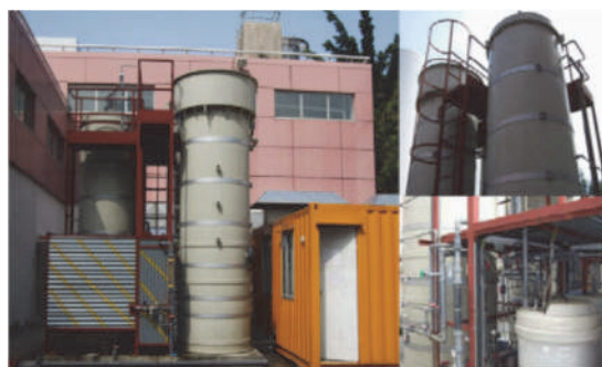
Figure 7.11 The SANI ® pilot plant at the Tung Chung Sewage Pumping Station (photo: HKUST).
