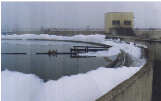
Figure 3.10 High concentrations of detergents create problems for a wastewater treatment plant operator (photo: M. Henze).
