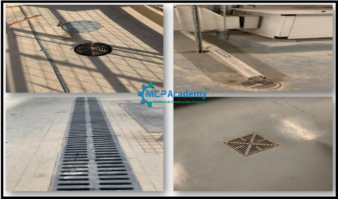
Roof Drain, Floor Drain, Channel Drain and Area Drain (PHOTO FROM SITE)
