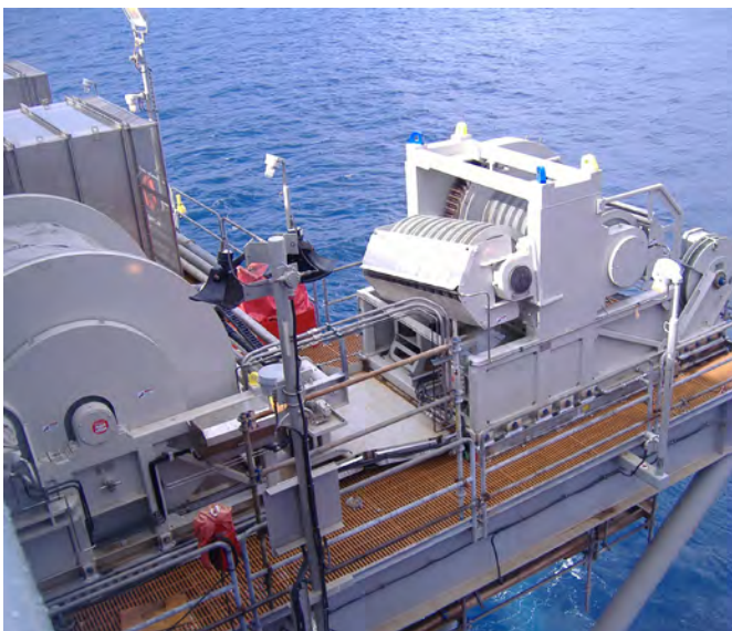
Figure 3. A custom-made, soft rope traction winch for Shell's Perdido platform was developed by Logan with many efficiencies in mind.
