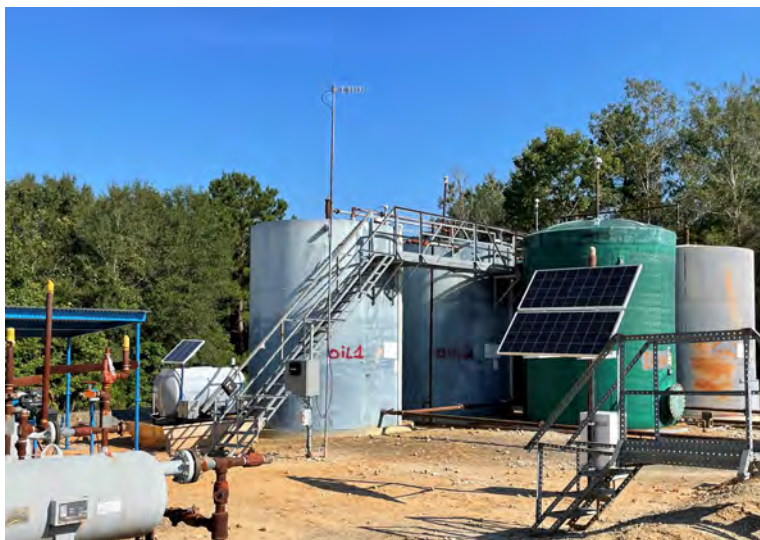
Figure 2. FreeWave provides solutions to a Faulconer Energy site.
