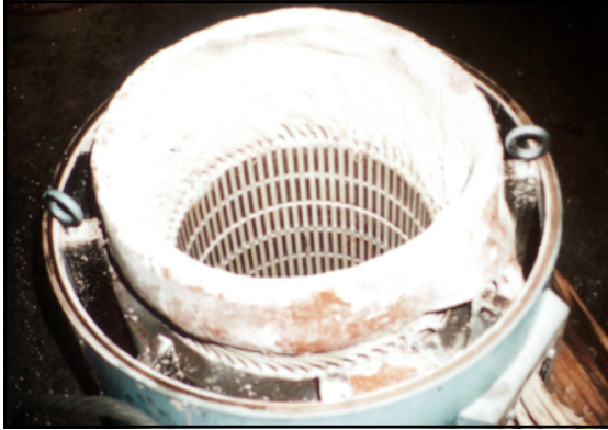
FIGURE 4: CLOGGED STATOR END TURNS AND VENT DUCTS
