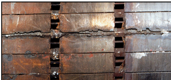
FIGURE 15: DAMAGE CAUSE BY ELECTROMAGNETIC EFFECT
