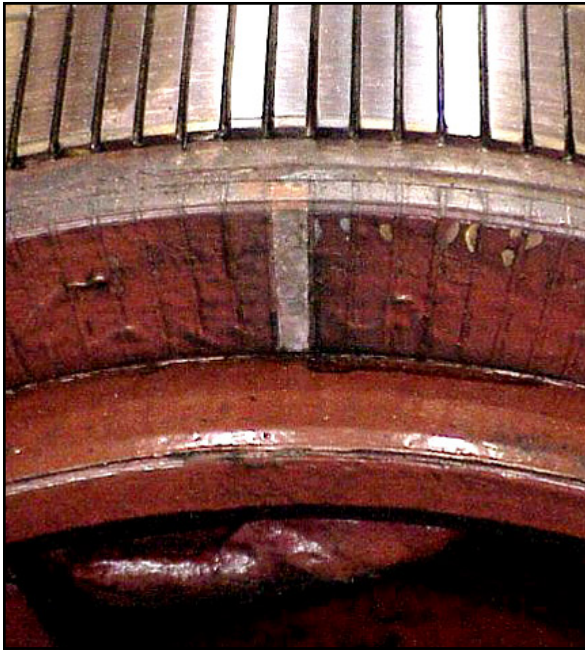
This banded commutator has an uncommon failure. Carbon or moisture trapped under the band has completed the circuit to ground of the affected bar.
