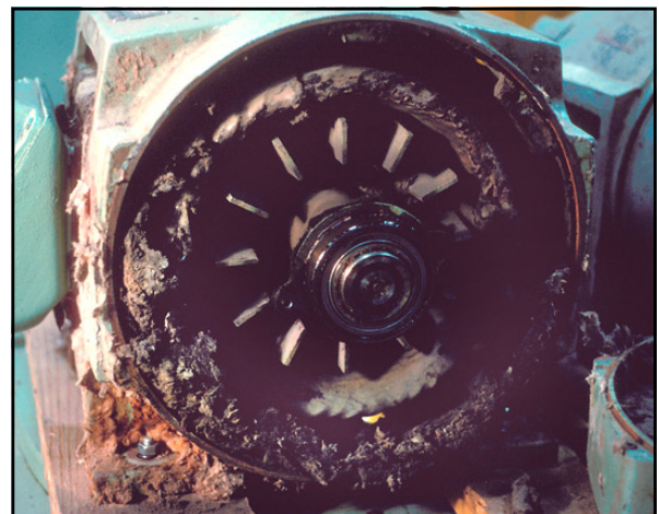
Moisture combined with foreign material can pack the windings or vent passages. This open motor is filled with pulp which restricts the flow of air. As a result, the winding overheated and failed.
