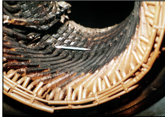
FIGURE 6: TRADITIONAL THERMAL OVERLOAD PATTERNS
