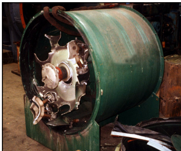
A foreign object entered the cooling air intake and damaged the blades of this fan.
