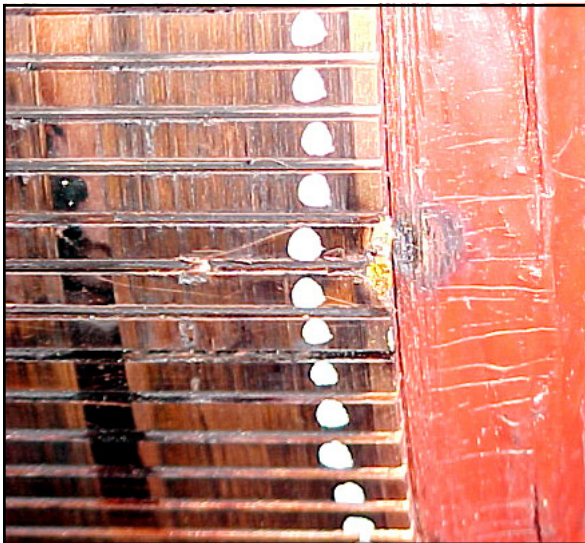
Shorted bars where copper melted.
