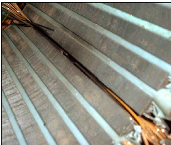
The conductor was improperly placed outside the cell wall/topstick so that it came into contact with the laminations resulting in a ground failure.
