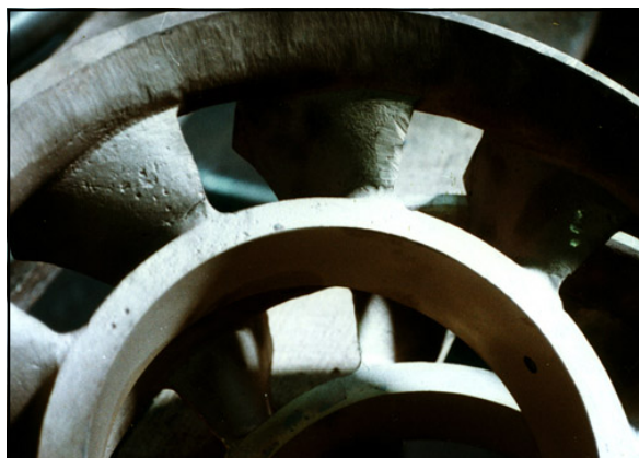
The blades on this unidirectional fan are being worn down by abrasion/corrosion.
