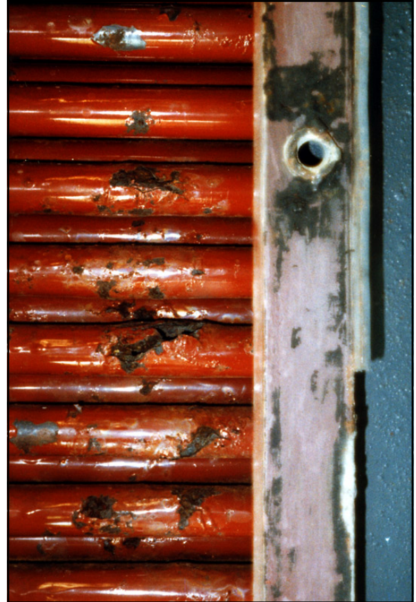
Cooling tube corrosion can occur inside or outside the tubes, wherever the atmosphere is most corrosive. Not only can the tubes leak, but oxidation is a thermal insulation.
