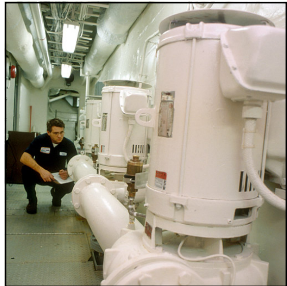
FIGURE 11: HORIZONTAL MOTOR MOUNTED VERTICALLY
