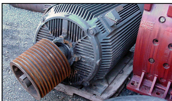
FIGURE 26: OVERTENSIONING OF BELTS
