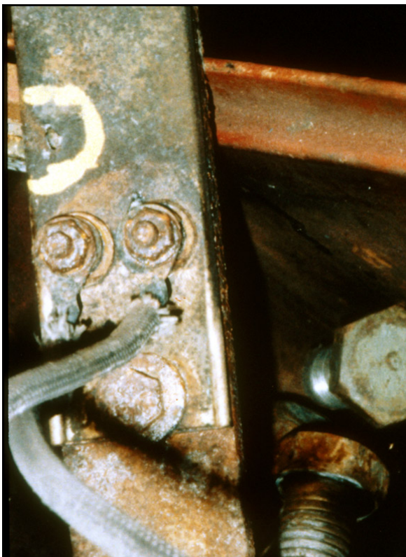
Thermal cycling of space heaters makes them susceptible to moisture and corrosion.
