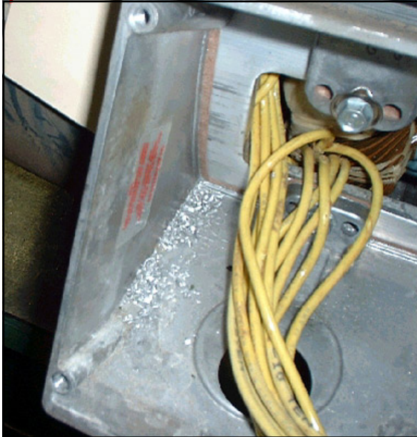
Foreign material: The conduit hole was drilled and filings were left in the terminal box.
