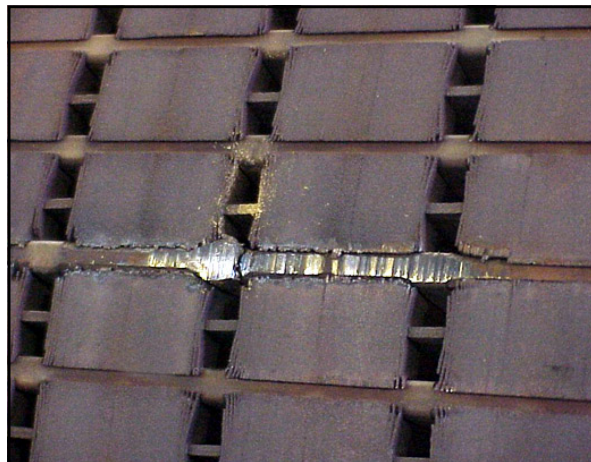
This loose bar was exposed due to severe vibration induced during a prolonged starting cycle.
