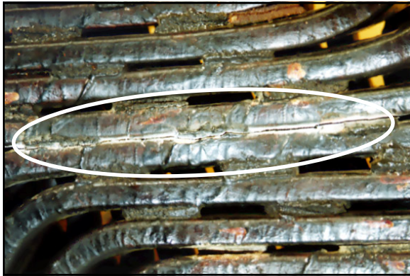
FIGURE 14: EXAMPLE OF PARTIAL DISCHARGE (CORONA)
